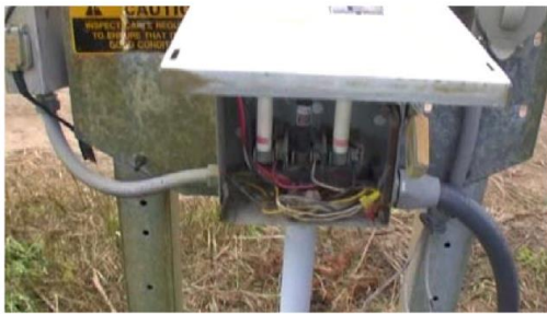
Figure 3. Power supply to Valley Pivot. Valley Pivot plugged into receptacle.
