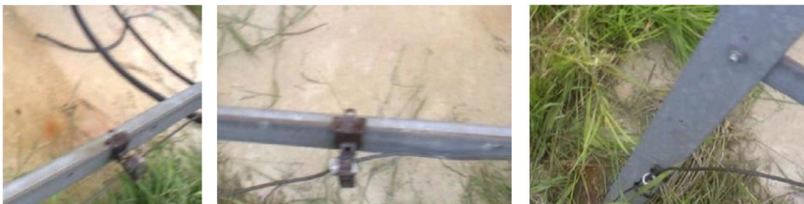
Figures 5-7. Path of Reinke ground wire.
