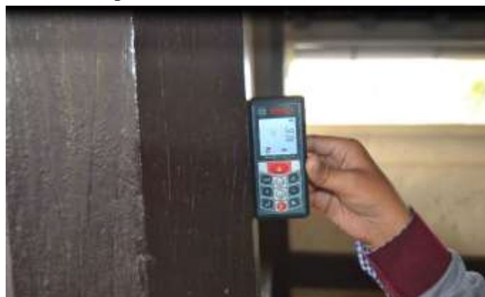
Figure 3. The Slope Measurement of The Mosque's Pillar (source: Putra, 2018)
