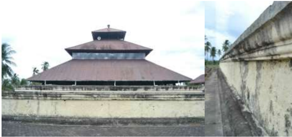
Figure 4. The View of The Mosque (left) and The Condition of The Mosque Walls (Right) (source: Putra, 2018)
